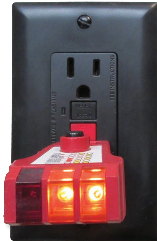
A GFI tester plugged into a GFI outlet.
