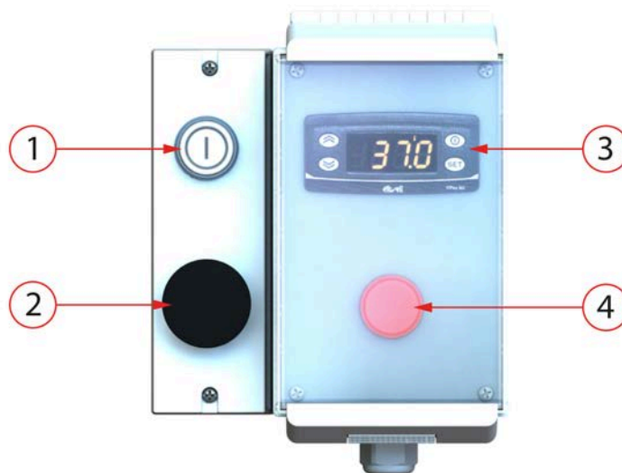
Figure 2: Overview of the control panel
